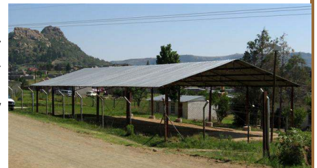
While we were in America, Bro. Marais and volunteers from the church erected the structure and welded it together. The next phase will be to pour a concrete floor.
