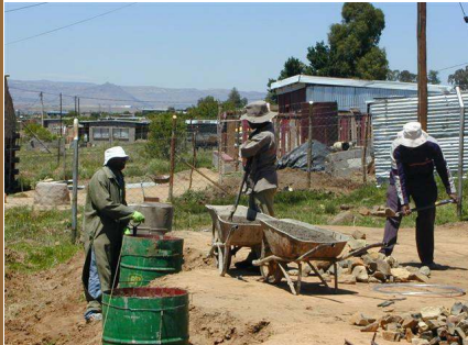
After several days of back-breaking pick and shovel work to level the site, we poured concrete pillars for each pole.
